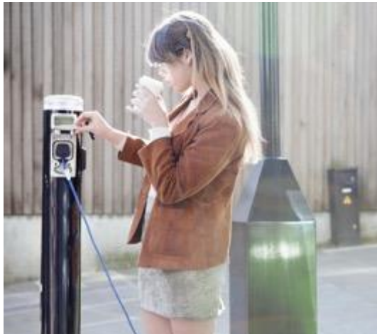
EV Charging Infrastructure
