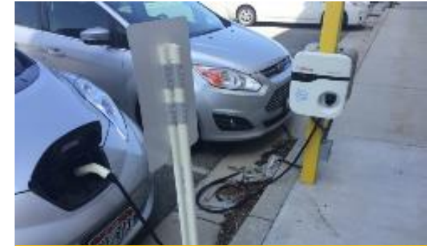
No cable damage
