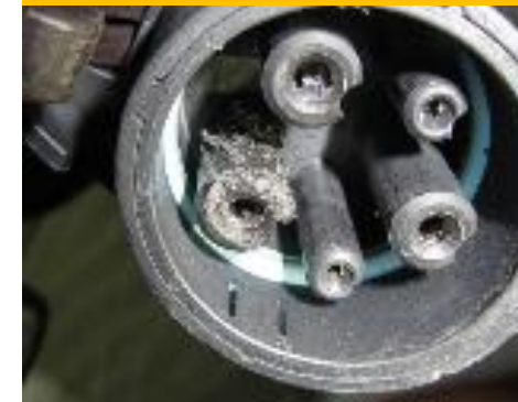
No connector failures
