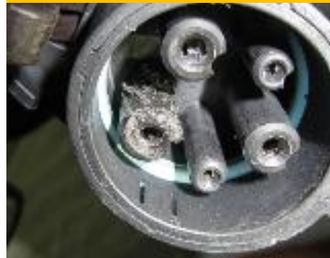
No connector failures
